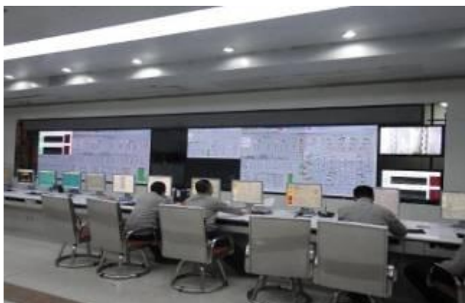
[Control Room] 2x4 Urumchi, China
